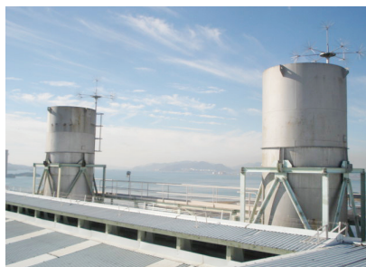
HOT Reheater Safety Silence
