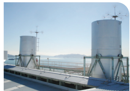
COLD Reheater Safety Silence
